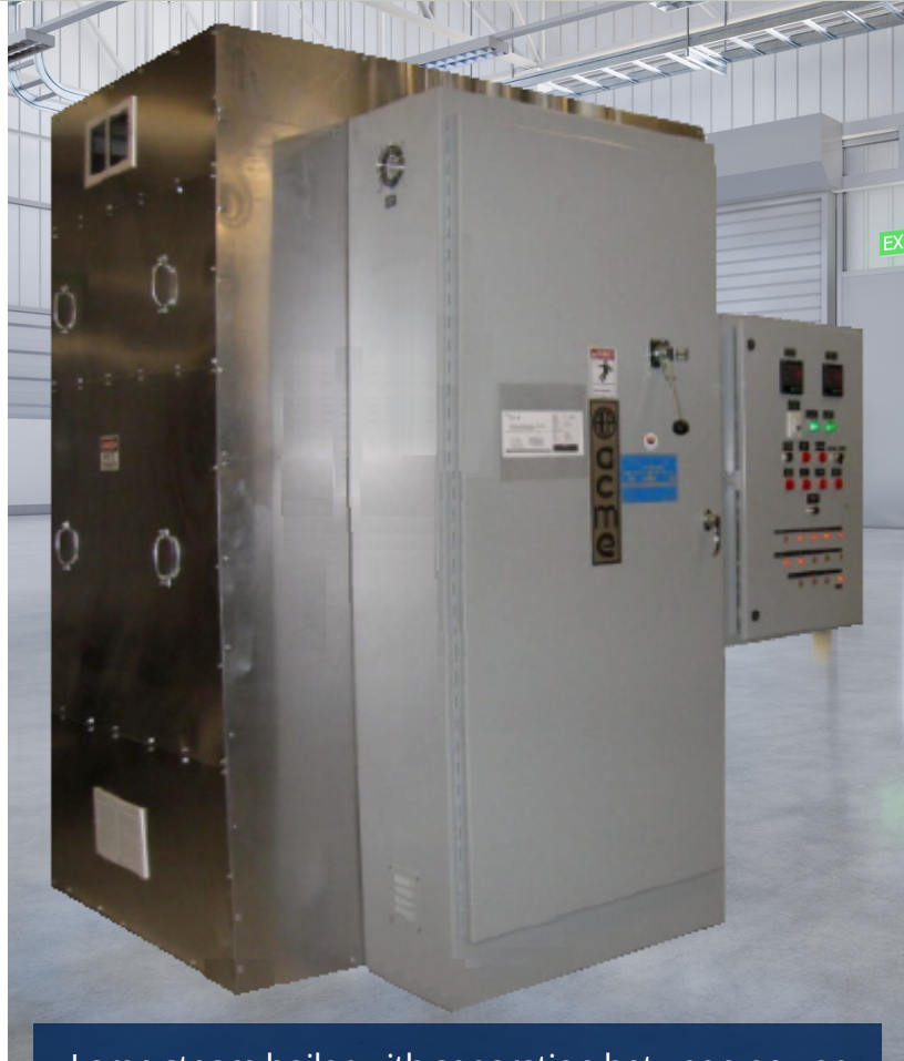
Large steam boiler with separation between power and control panel
