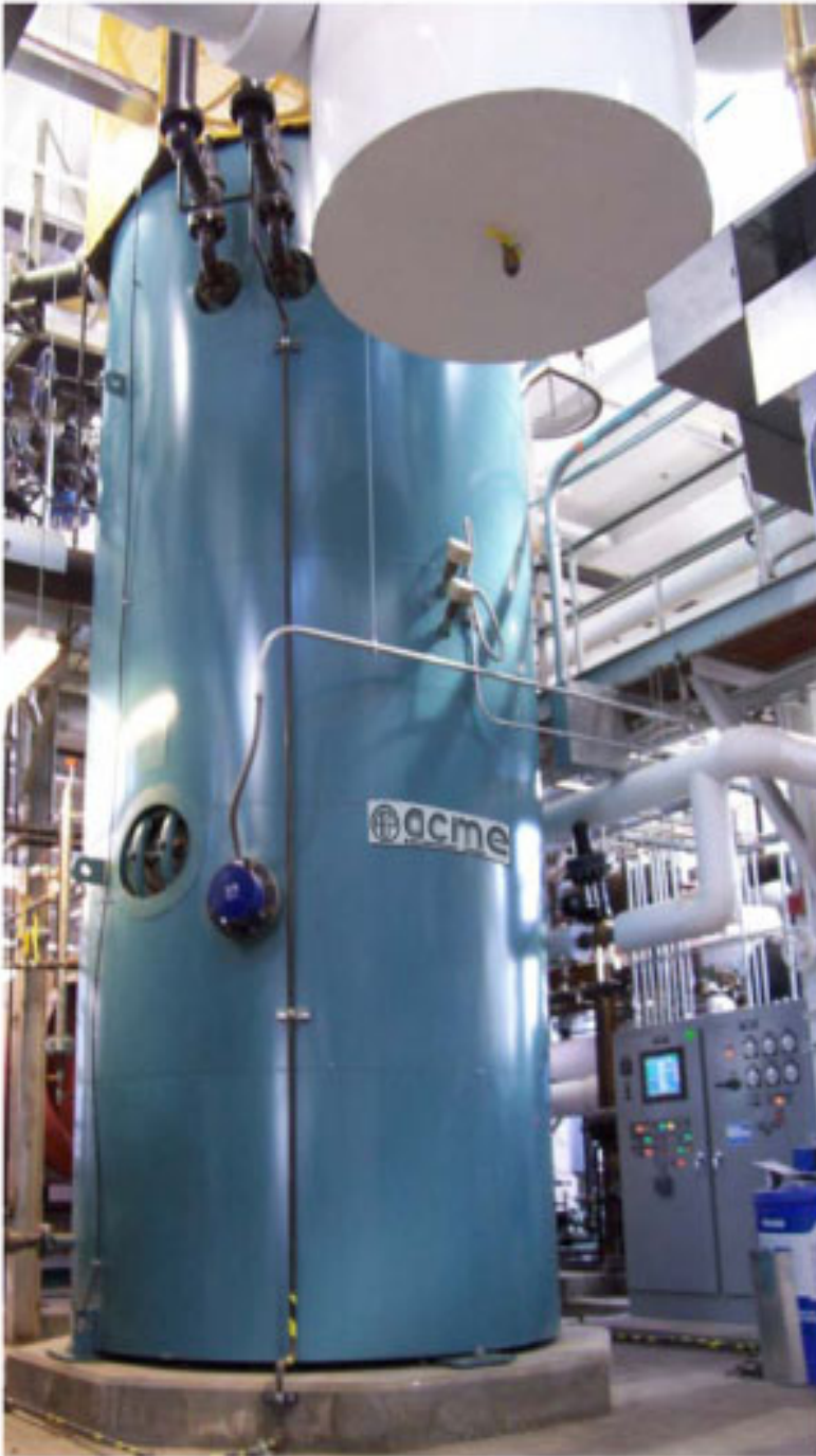
CEJS HIGH VOLTAGE ELECTRODE BOILER INSTALLATION WITH CONTROL PANEL IN THE BACKGROUND
